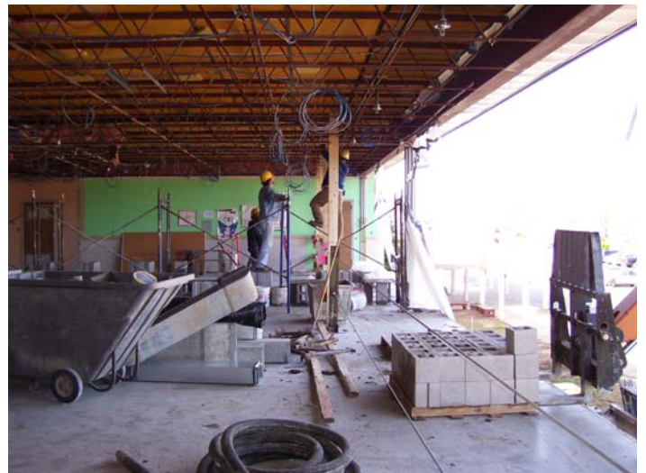
Renovation of existing building, exterior wall demolished to be replaced with new high performance exterior envelope.
